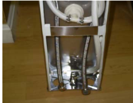
Cold & Hot Pipes
